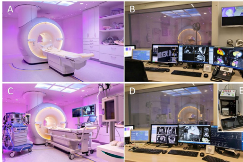
FIGURE 1 Full transformation of the pre-existing MRI environment (A,B) into an interventional cardiac MRI suite (C,D,E)
